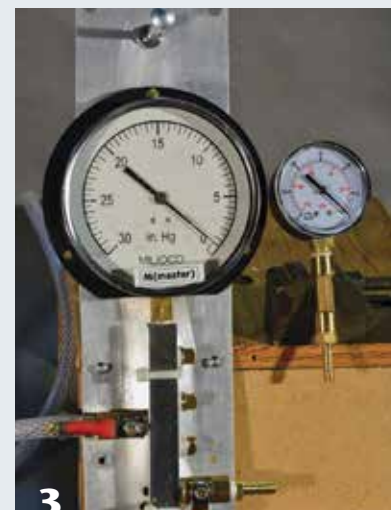
When running airflow tests, use a large vacuum gauge like the one pictured left. The smaller one is an inexpensive unit commonly used in vacuum systems and may not deliver sufficient accuracy and readability. Also, inexpensive gauges may not be accurately calibrated, leading to differences in the readings when using more than one gauge. For consistent measurements, gently tap the gauge before each reading to help overcome internal friction of the needle mechanism.
