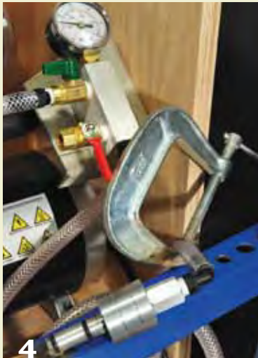
4 A C clamp is being used to temporarily close off the tubing to isolate the rotary coupling from the rest of the system.
