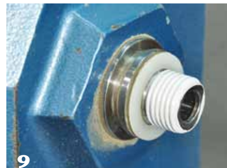
For this system, it was found that using Teflon thread sealing tape on the spindle significantly reduced the leakage.
